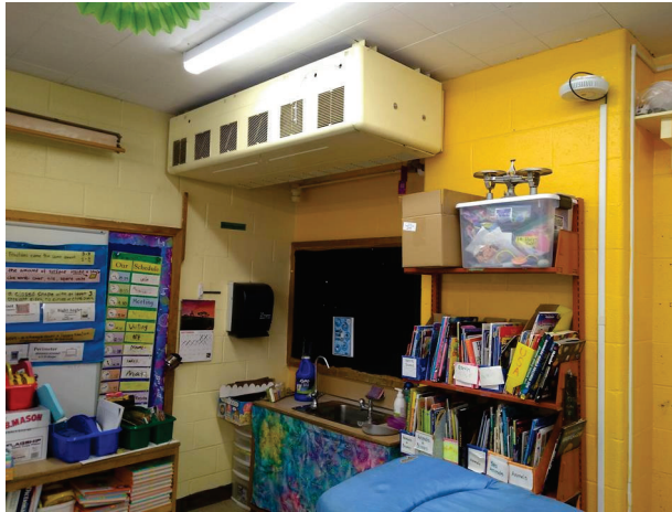
20. Classrooms have outdated and inefficient unit ventilators.
