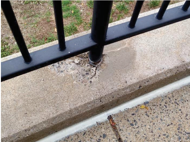
1. Concrete has spalled at some rail posts.
