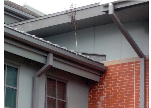
3. Some gutters are clogged with vegetation.
