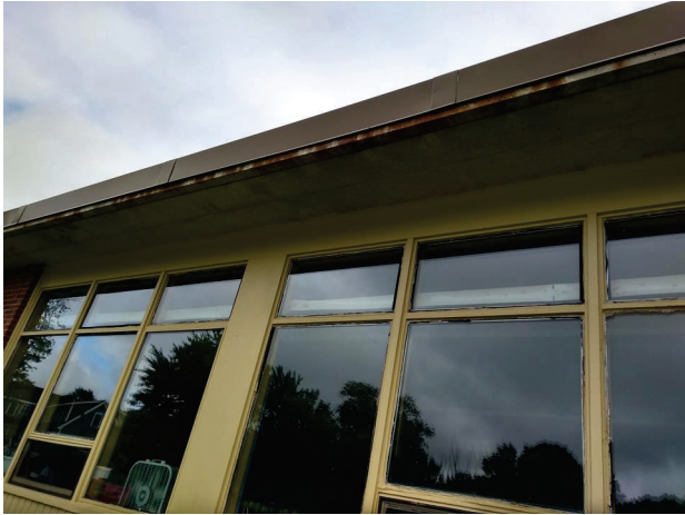
7. Original roof soffits have corroded.
