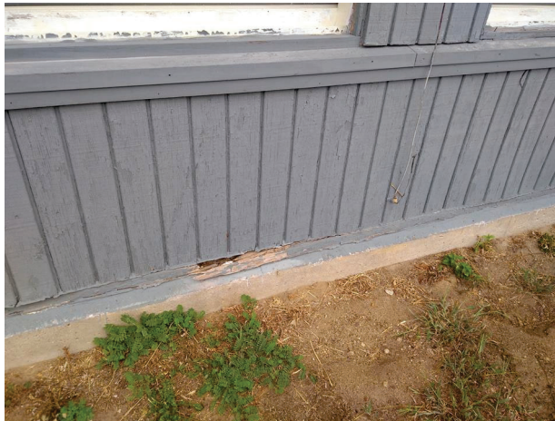
5. The wood siding is rotted and damaged.
