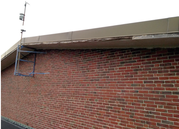
13. The fascia is rotted at the Cafetorium.
