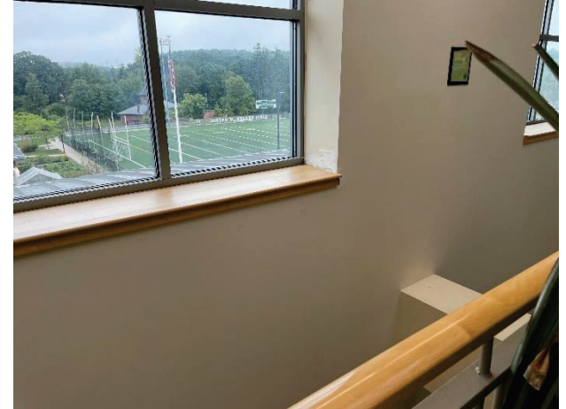
9. Several windows show signs of water damage.
