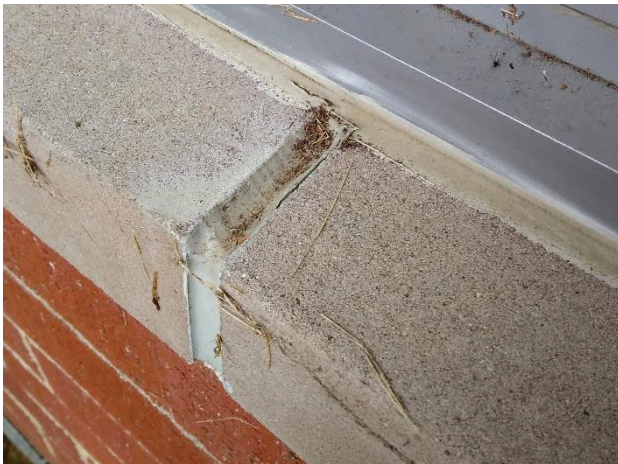
4. Some sealant shows early signs of deterioration.
