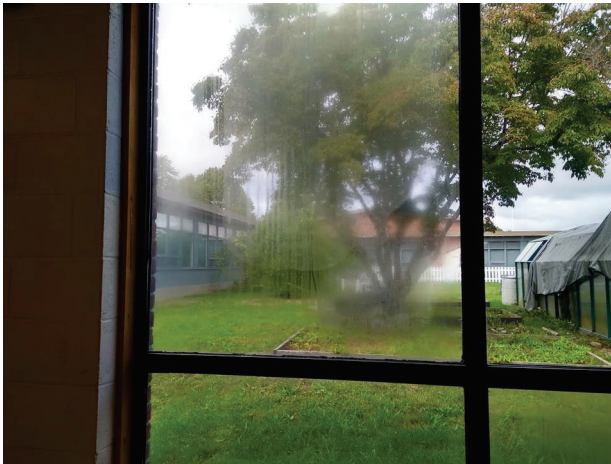
4. Thermal pane window has seal failure.
