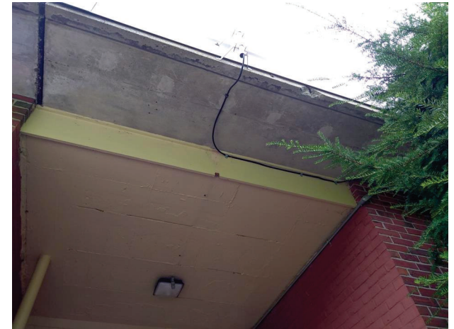
6. The concrete facias and soffits have spalled.
