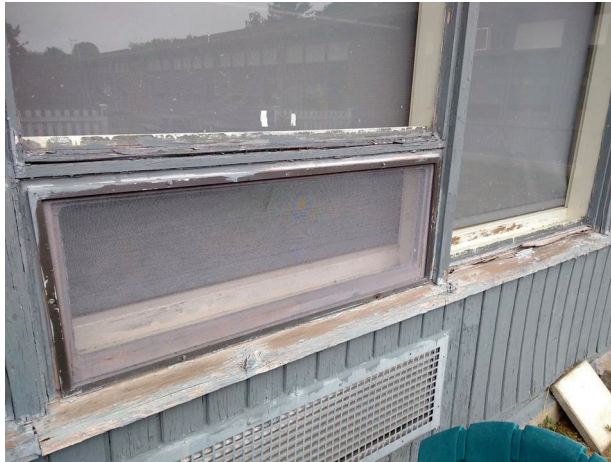
2. Original windows and trim have deteriorated.
